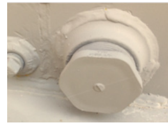
Clean out port and internal hydraulic spill reservoir
